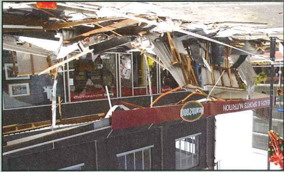
CBD of Gisborne after the earthquake.
