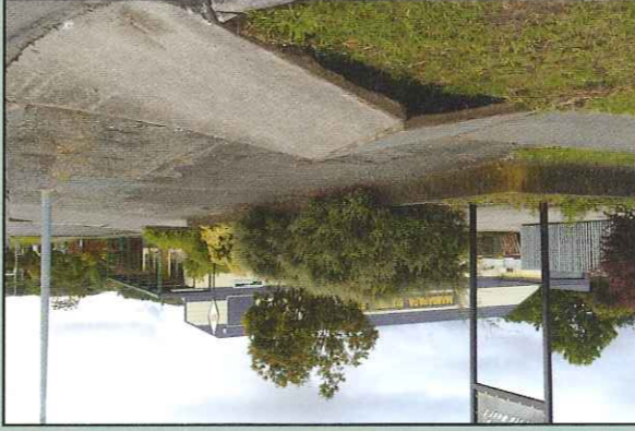
Damage to roading due to the earthquake.
